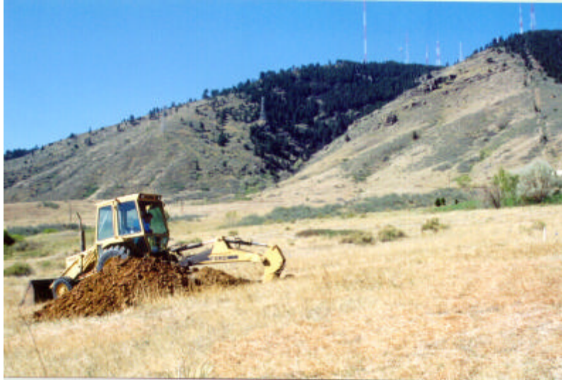
Figure A.2. Photograph of Backhoe Test Pit #1, looking southwest (see Figure 2 for location).
